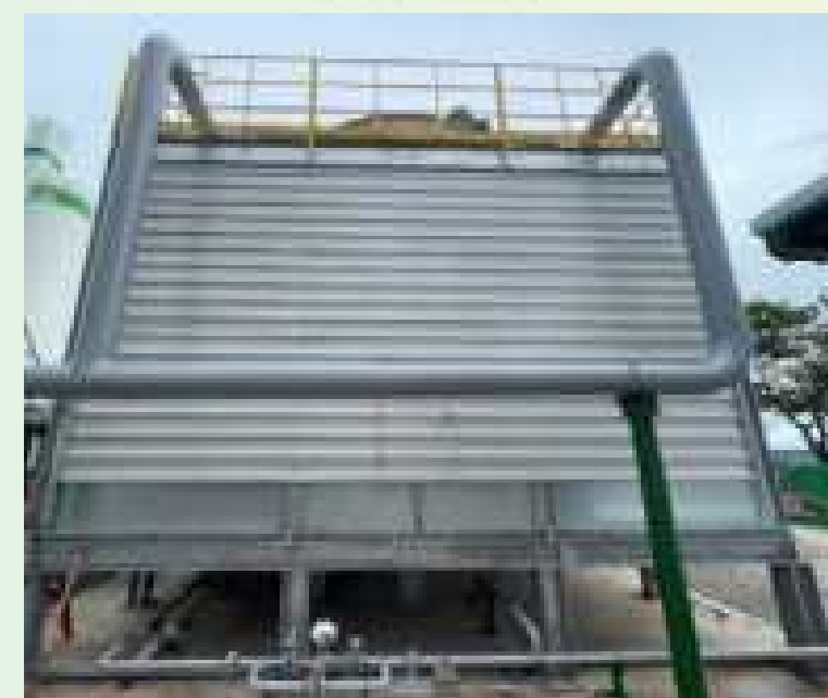
New Package Cooling Tower
