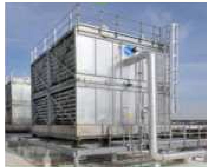
Open Cooling Tower
