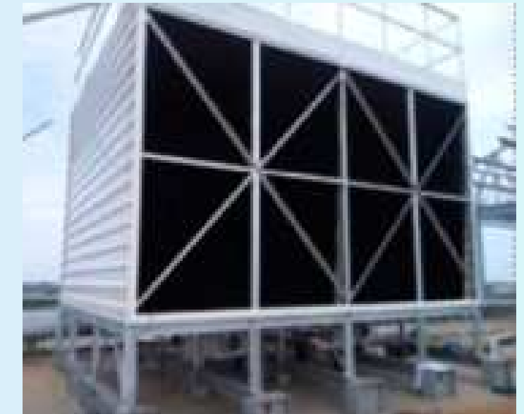
New Package Cooling Tower
